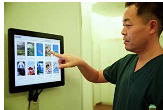
Staff use smartphone-style touchscreen controls to choose themes. Dynamic lighting, wall projection, ceiling displays and sound create a relaxing environment
